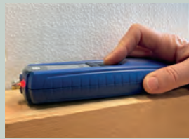
Non-destructive measurement by means of a single-point contact area [LED flashing for limit exceedance]
